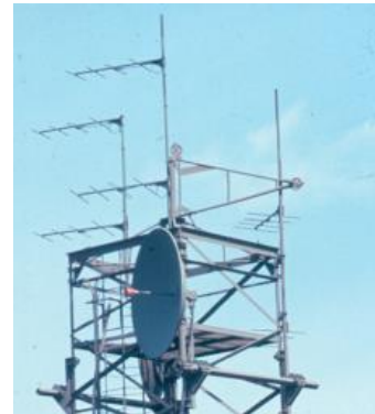
Figur 19: Yagiantenner (Foto: Aerotech Telub/Arboga)
