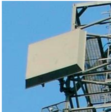
Figur 18: Dipolantenn (Foto: Michael Grund, FMV)
